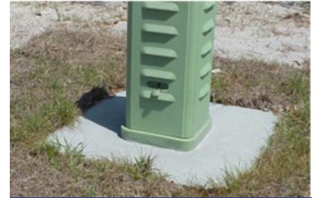
Air Release Valve
